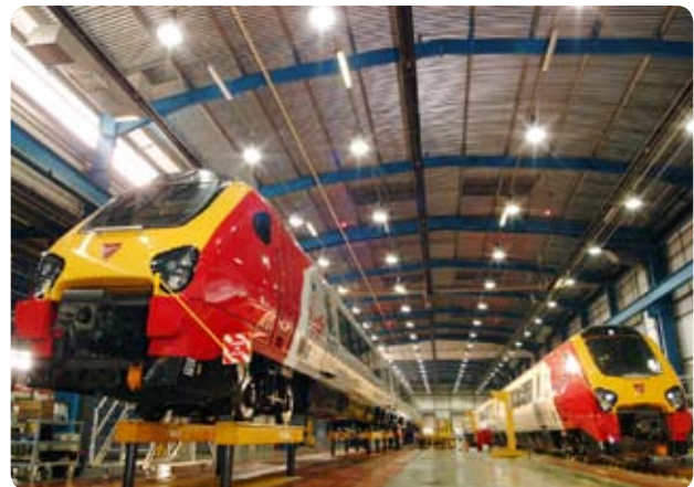
Continuous radiant tube heaters along the length of a large building
