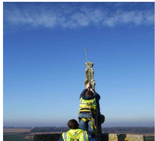
Workman repairing the lightning conductor on the 132 feet tower of Winterton Parish Church. The photograph was taken by Sandra Laws, Church Warden, on a cold November day.
