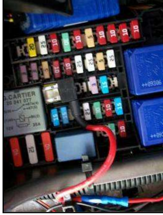
Fuse box for ignition sense.
