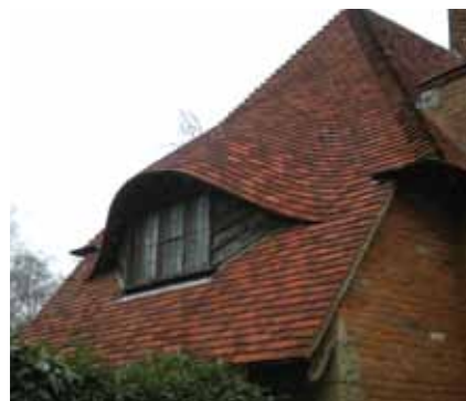
Front cover: The NFRC gold award-winning Sussex Cottage, whose roof was renovated and refurbished by Clarke Roofing Southern Ltd
