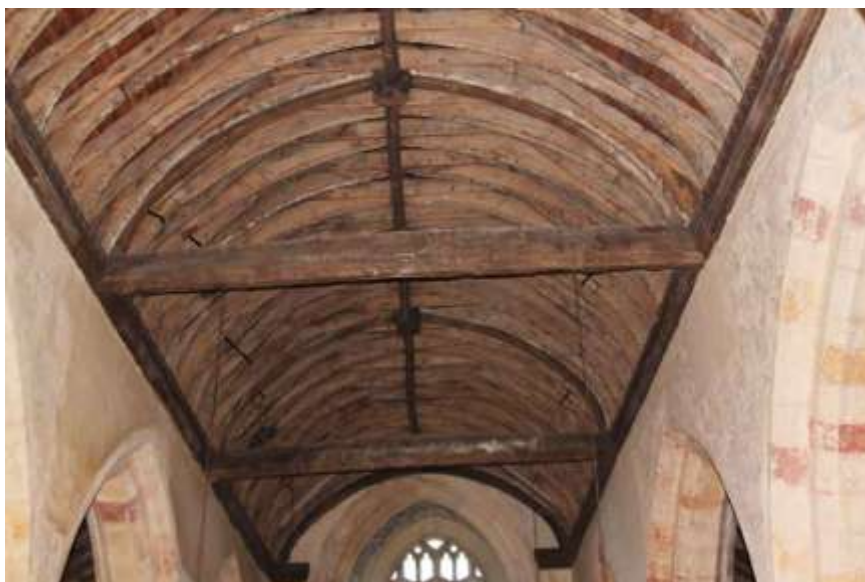
Three-bay late medieval arch-braced collar rafter roof in the Church of St. Giles, Imber
